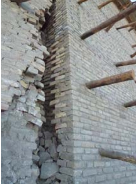
Fig. 6 Retaining wall was reinforced by horizontal wooden logs
