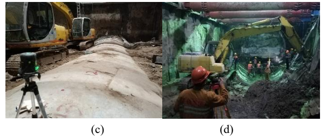
Fig. 4 Damage and repair process of shield tunnel accident (a) groundwater and soil gushing into the tunnel, (b) segments settling and misplacement, (c) tunnel settlement, (d) excavation of the damaged tunnel
