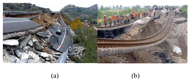
Fig. 36 Photo of the embankment failure in (a) Luochang highway and (b) Railway subgrade
