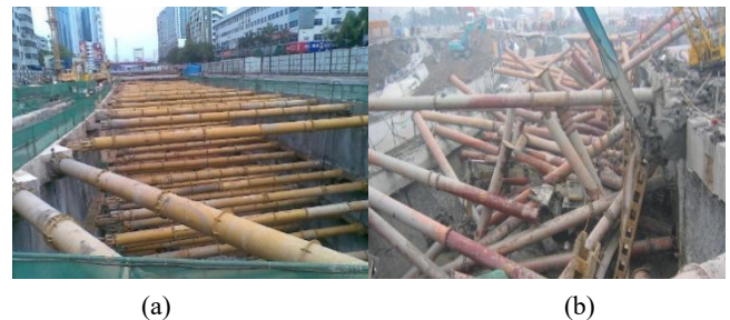
Fig. 14 Retaining system of deep excavation and its failure at Xianghu Station of Hangzhou Metro Line 1 (a) Excavation retaining system (b) Failure scene of the retaining system
