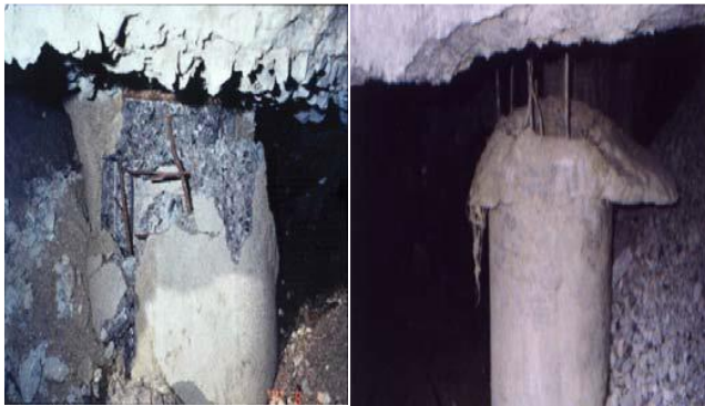
(a) Bending failure (b) Pull out to destroy
