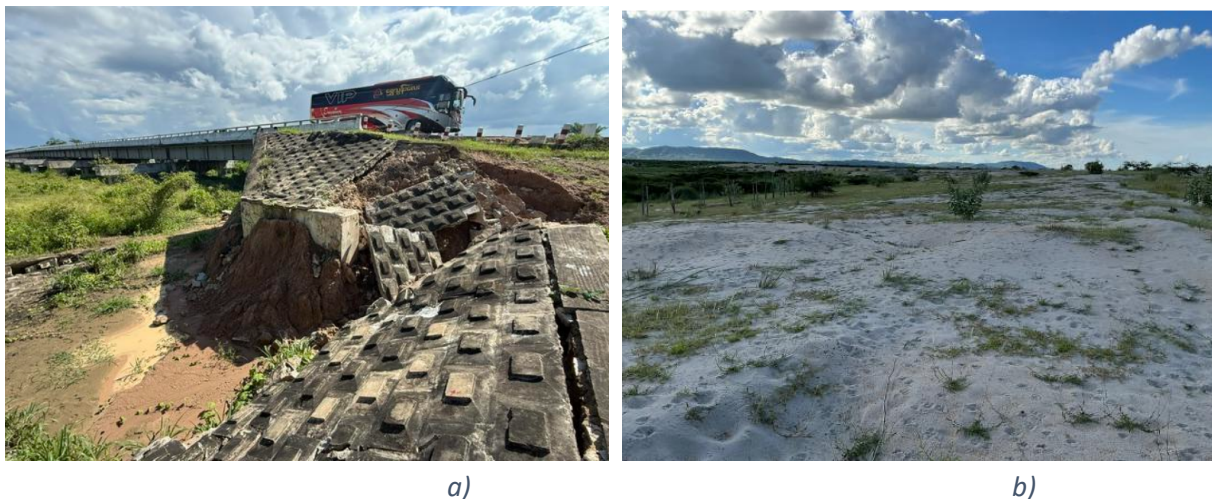
Figure 8. a) Abutment damage along the Yangon – Mandalay highway; b) sand boils at shopping mall site, Mandalay.
