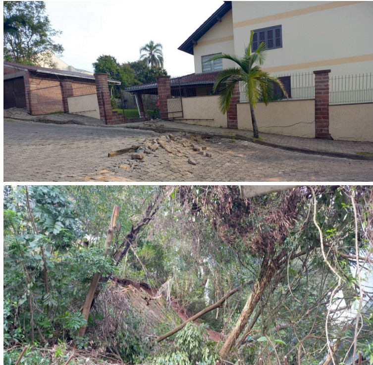
Figure 6. Cracks in streets and instability suggesting large scale ground failure.
