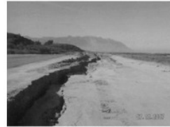
Crack and settlement (Athens-Thessaloniki highway)
