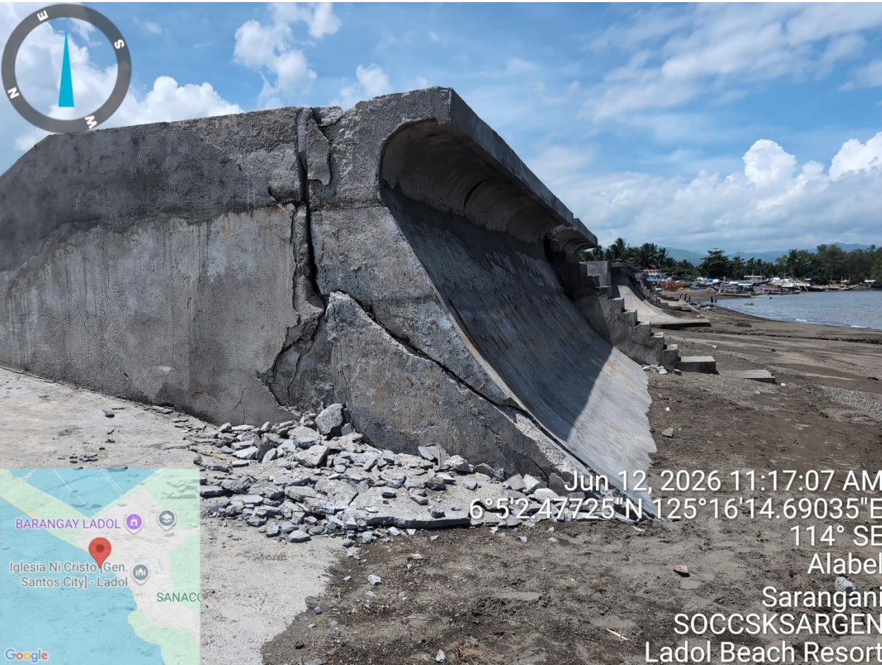
Damaged Sea wall in Ladol Beach, Alabel, Sarangani
