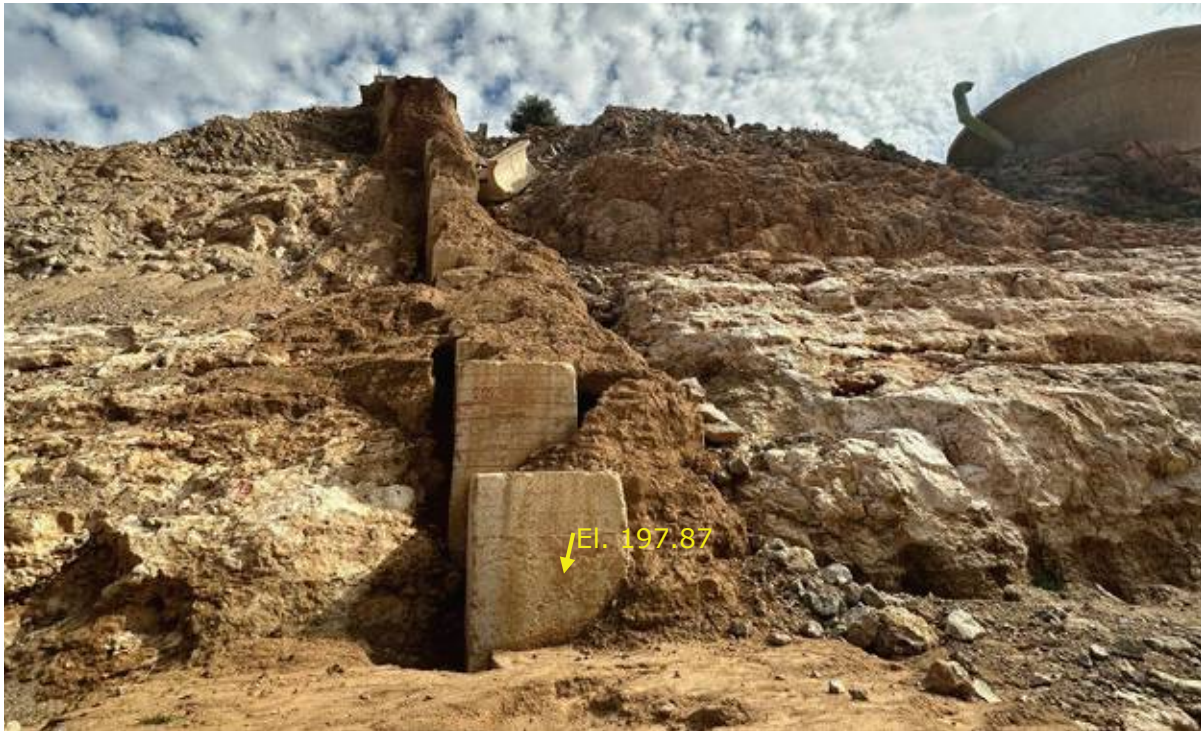
PHOTO 4.2. View of the right abutment of the Abu Mansour Dam where the embankment was totally washed away. Concrete blocks correspond to the centerline of the core foundation and the grout curtain drilling.
