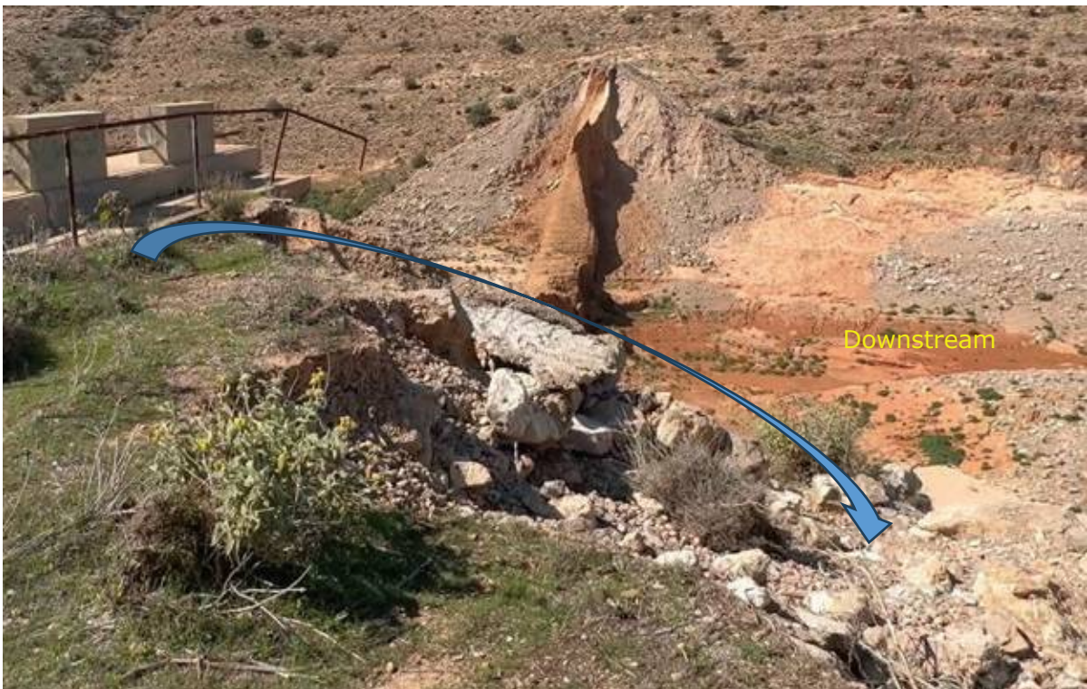
PHOTO 4.1. Erosion due to the water overflowing the right abutment of the Abu Mansour Dam.
