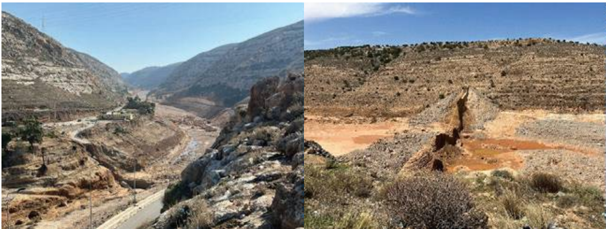
PHOTO 4.8. Remains of clay core in collapsed dams: the Abu Mansour Dam (left) and the Derna Dam (right).
