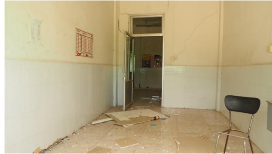
(d) The same building ten meters away from the fault (leftward in (b))
