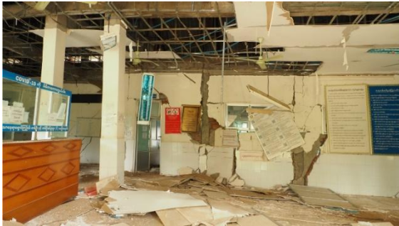
(c) Damage inside the main building
