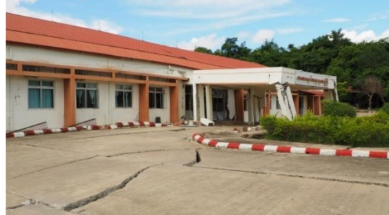
(b) Main building resting directly on the fault dislocation
