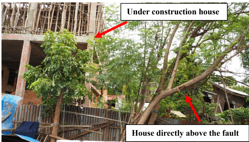
Photo 14: Contrast of damage of two adjacent houses on the opposite side of fault dislocation in Photo 12
