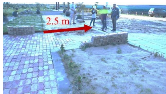
Photo 13: Fault dislocation in a solar power station
