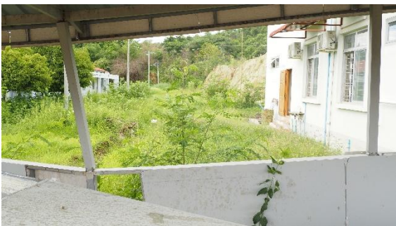
(e) Continuation of fault rupture on the northern side of the site
