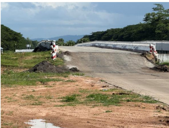
Photo 1: Liquefaction induced damage to road
