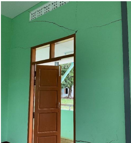
Photo 8: Damage to school buildings
