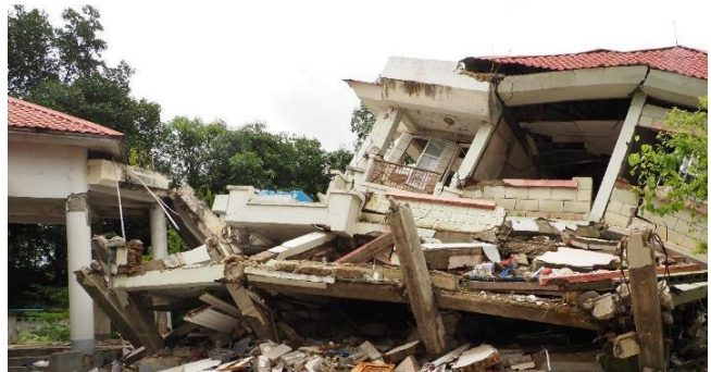
Photo 11: Structural damages in lower storeys of buildings (Nyaung Pin Gyi Su)
