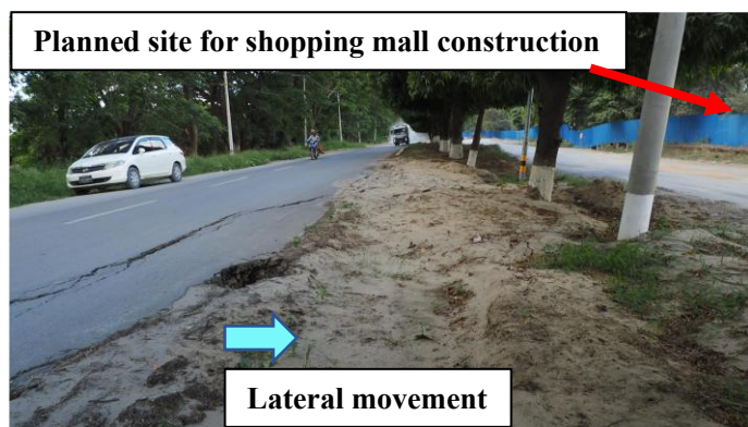
Photo 4: Liquefaction-induced damage to the nearby road surface
