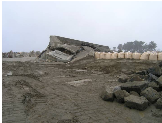
Fig. 13 Destroyed sea wall near Abukuma River mouth
