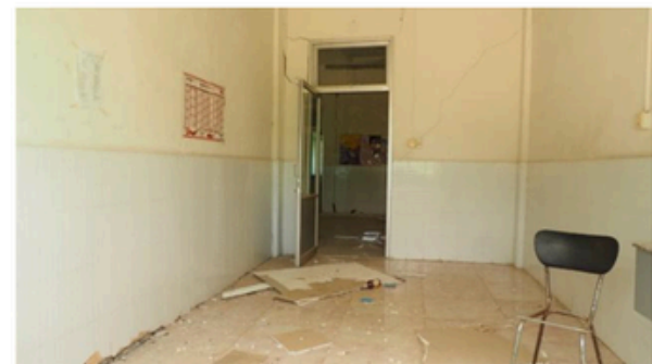
(d) The same building ten meters away from the fault (leftward in (b))
