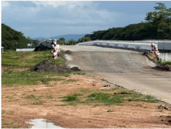
Photo 1: Liquefaction induced damage to road
