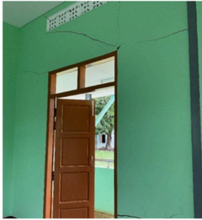
Photo 8: Damage to school buildings
