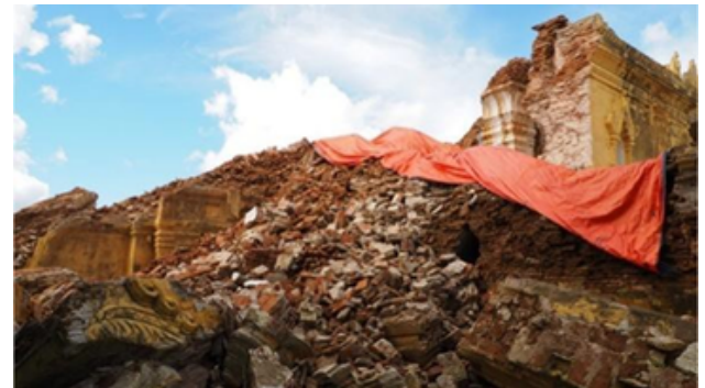
Photo 16: Destroyed Me Nu Brick Monastery in Inwa
