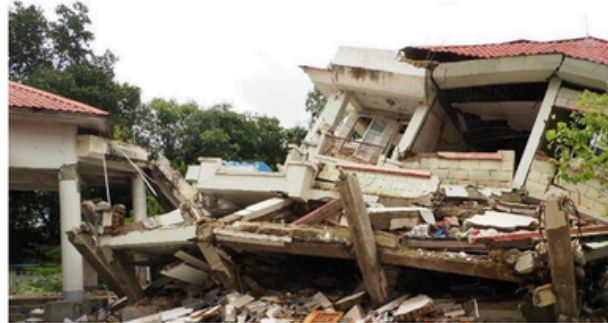
Photo 11: Structural damages in lower storeys of buildings (Nepyidaw)
