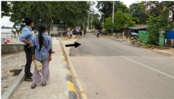
Photo 12: Right-lateral fault dislocation in Sagaing (Left bank of the Ayeyarwady River, near Mandalay)
