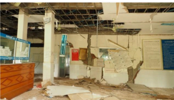
(c) Damage inside the main building
