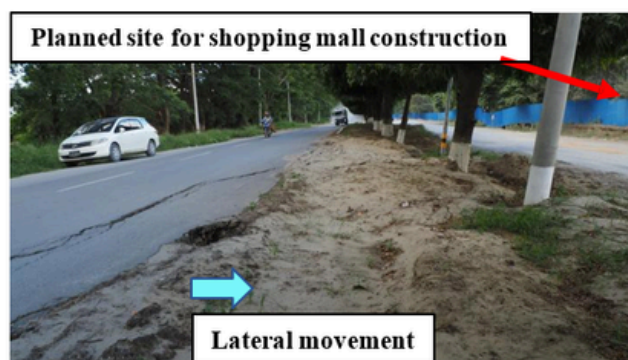
Photo 4: Liquefaction-induced damage to the nearby road surface
