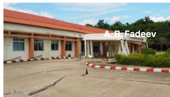
(b) Main building resting directly on the fault dislocation
