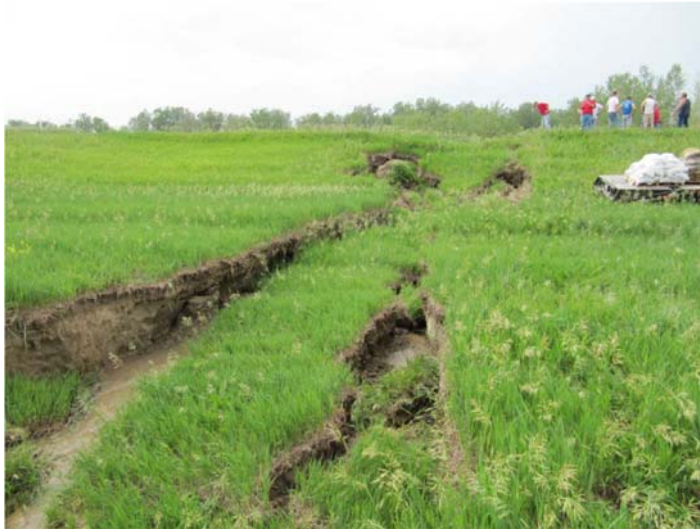
Figure 3.13 The initial distress in the levee L-575.
