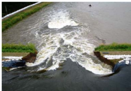
Figure 3.10 Breach occurring (taken around 0700 hr, 27 June 2008).
