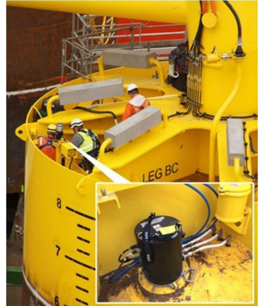
SHM system for a SBJ. Photo: NGI
