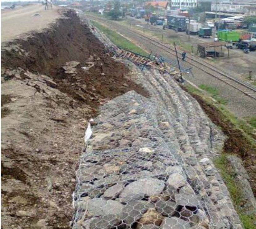
Figure 3. Local failure at the critical section along the railway and main road.
