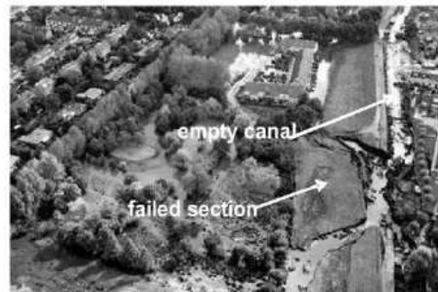
Fig. 1. Failed canal dike at Wilnis, August 2003.
