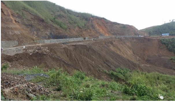
Figure 1. Typical retaining wall failure along major roads.
