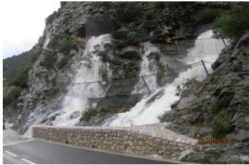
Figure 16. Safety problems due to stone falling in the road N-621 after intense rains. Situation of PK 158,140 MI produced by heavy rains on rocky slope (upstream) performed the performance.
