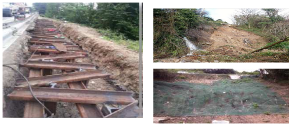
Figure 15. Lane swelling, laying of geogrid, bolted cable network and reconstruction of water trough on the N-629 road caused by heavy rains.
