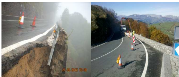
Figure 16. Subsidence of the N-629 road platform caused by heavy rains and provisional signposting
