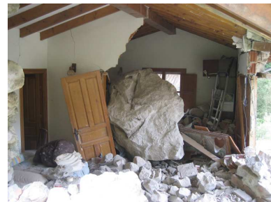
Figure 2 Situation in the road N-621 produced after intense rains with stone falling.
