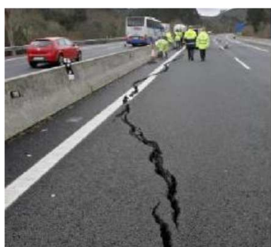
Figure 5 Cracking of the road way with descent of 100 cm in the A-8, Liendo.
