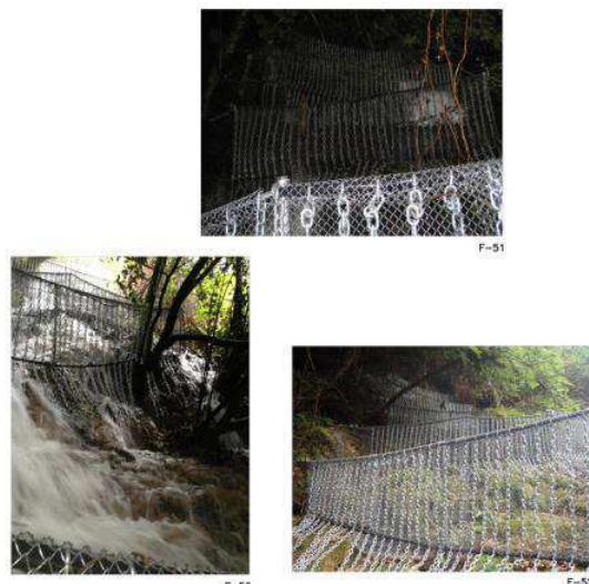
Figure 9. Situation of the PK 169,050 MI produced by rains. Protection channels 2, 3 y 4.
