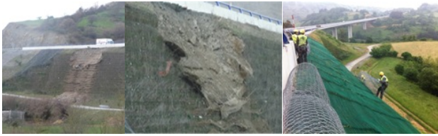
Figure 14. Safety problems due to stone falling in the road N-621 after intense rains.
