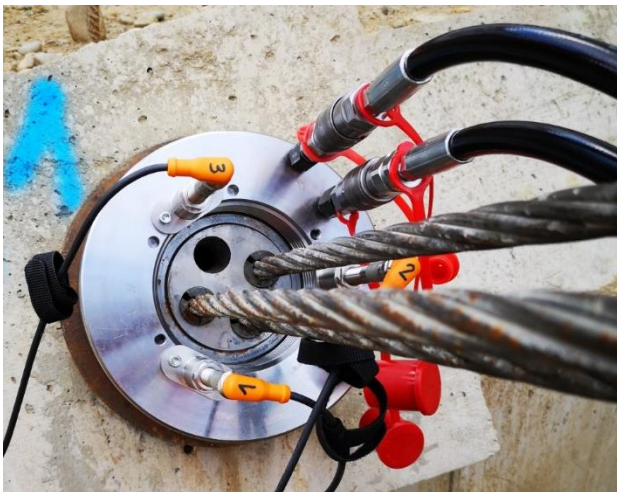
Figure 10. Testing equipment with additional installed displacement sensors (orange caps) in the field tests
