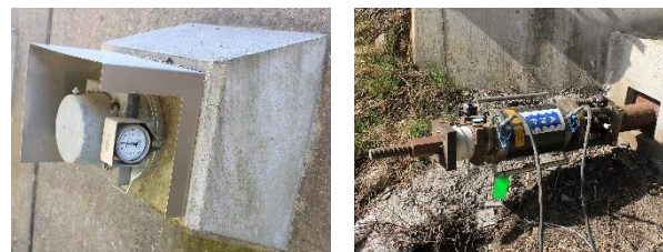
Figure 3. Determination of the anchor load during service life, anchor load cell (left), lock-off-test on an anchor (right)
