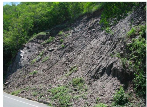
(b) Weathered rock slope failure at Km 66+900
