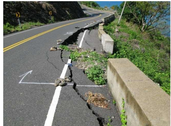
(a) Fill slope failure at Km 66+900
