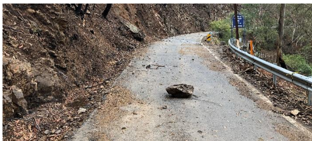
Figure 10. Rockfall from the upper natural slopes above Five Mile Hill
