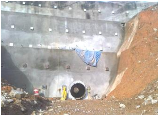
Figure 11. Combination of Estatec System with microtunnelling techniques
