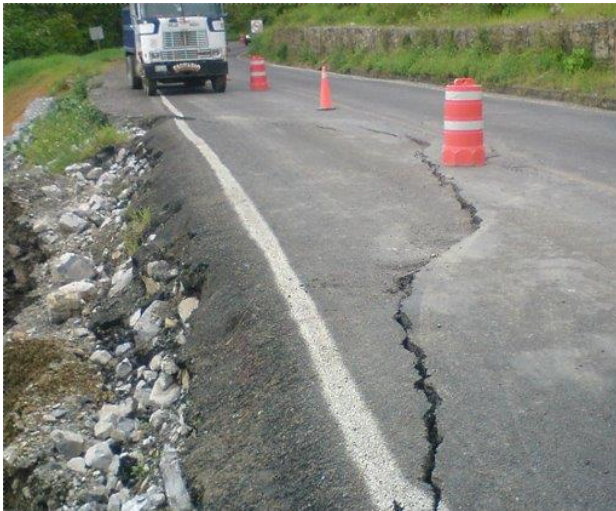
Figure 2. Pachuca – Tuxpan Road, Km 105+200. It's observed cracks on the top of the rotational movement
