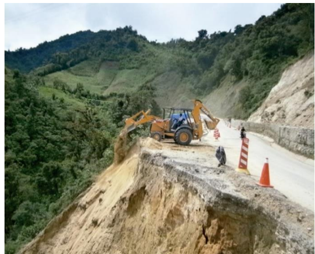
Figure 8. Landslide Km 46+130 Huixtla – Motozintla road.
