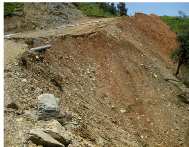
Figure 4. Case 2. Km 2+720 Zoquital – Catalina pipeline. Rotational landslide and regressive erosion.
