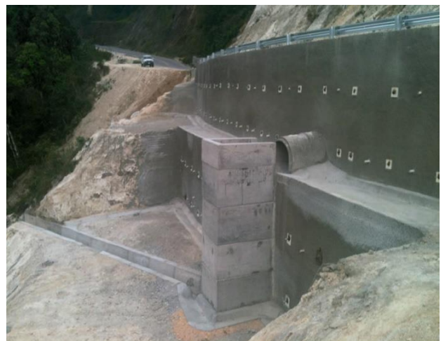
Figure 9. Landslide Km 46+130 Huixtla – Motozintla road.
