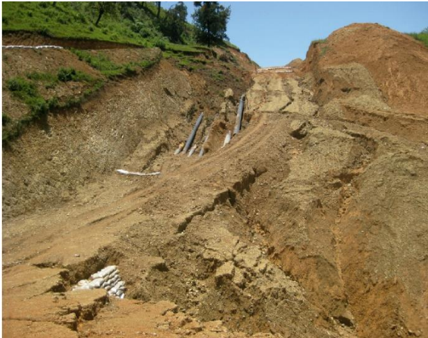
Figure 6. Km 2+600 Zoquital – Catalina pipeline. Landslide and regressive erosion.
