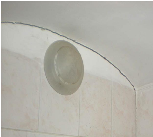
Figure 4. – Cracks within the building at Michurina St., 15 (the south wing)
