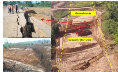
Figure 2. 1 st ground cracks observed during culvert excavation (24 Feb 2017). Yellow dashed lines indicate the design road alignment.
