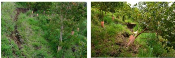
Figure 7. Areal view of the landslide area (28/10/2017)
