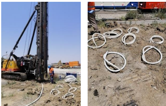
Figure 10. Installation of conventional circular PVDs at a field site for testing the VWM (left), and installed drains in a grid of seven drains.
