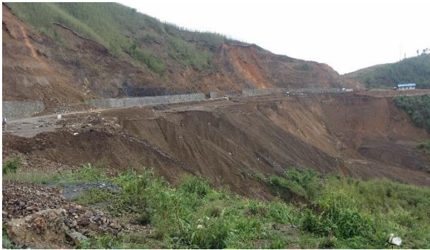
Figure 1. Typical retaining wall failure along major roads.
