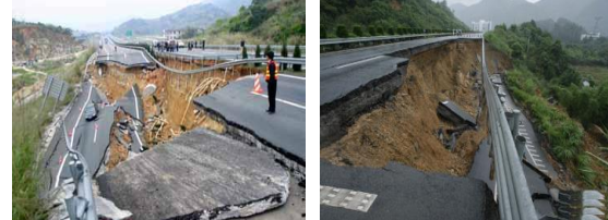
Figure 15. Failures case histories of embankments
