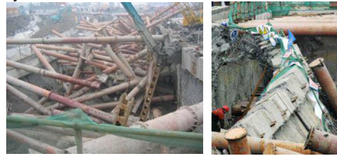
Figure 7. The messy struts after the collapse
