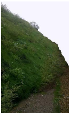
Figure 5. View of toe bulge.
