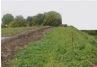
Figure 4. View of back-scarp.
