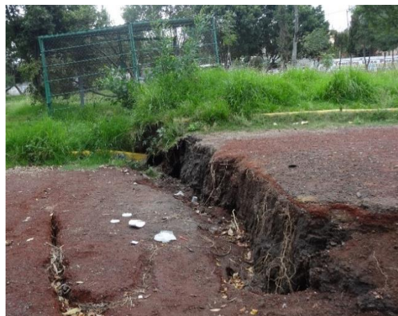
Figure 1. Activation of a pre-existing crack during the earthquake of September 19, 2017 (Deportivo Cananea, Alcaldía Iztapalapa).
