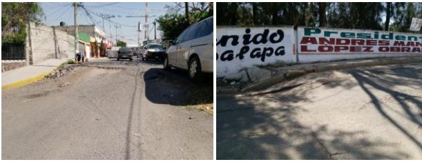
Figure 17. Examples of crack with step on streets in Iztapalapa municipality.
