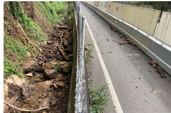
Photo 5: Rock debris accumulated behind concrete barrier at left and some over-topping evident against the temporary barrier at right observed on 24 March 2021 following high intensity rainfall
