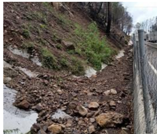
Photo 4: Erosion against barrier following 256mm of rainfall over 3 days in January 2020
