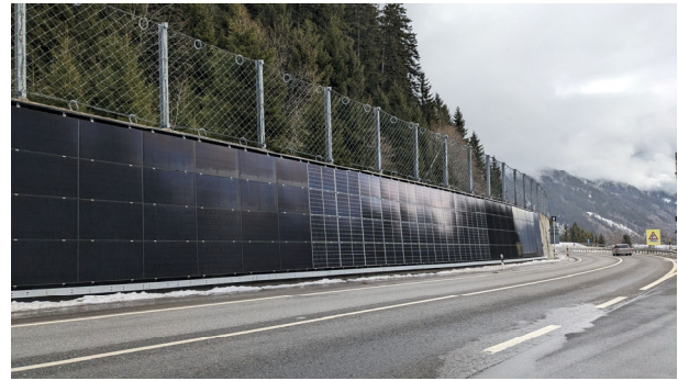
Figure 14. Photovoltaic pilot installation that follows the shape of the structure, with panels of different frame colors grouped together and parallel to the road. Picture: PPIC.
