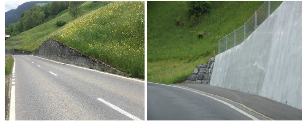
Figure 7. Left: good connection at the ground level; right: Example of a wall that was too short and was extended in an unattractive manner. (Canton of Bern, 2023)
