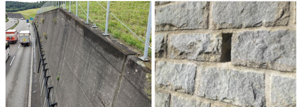
Figure 12. Left: retrofitted drainage system, with exposed piping and unsightly limescale deposits. Picture: PPIC. Right: a good example of drainage perpendicular to the wall via a vertical opening (Canton of Bern, 2023)
