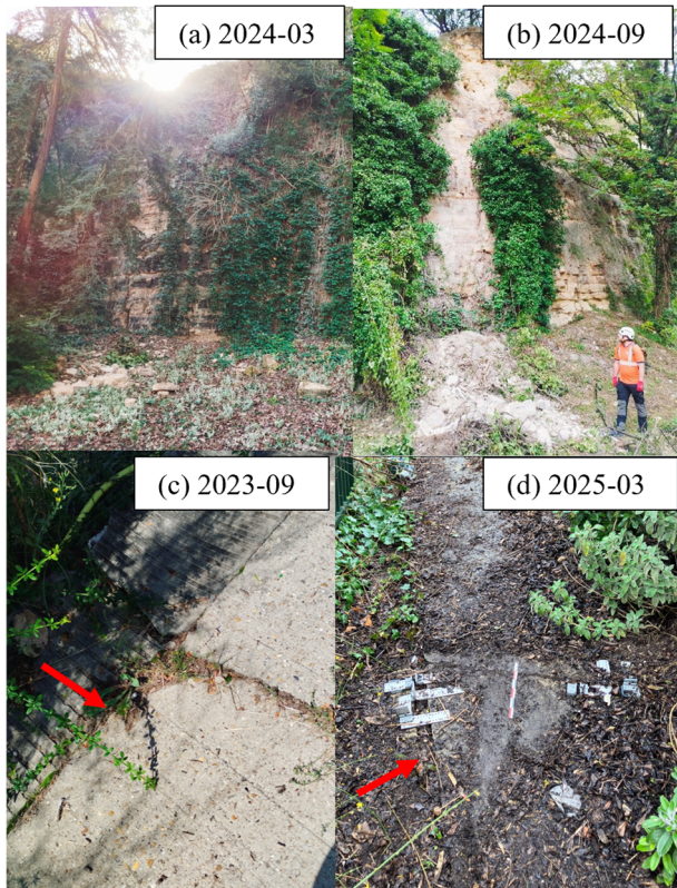
Figure 4. Observations during field visits. Top: examples of rockfalls. Bottom: Pathway photographed in September 2023 and March 2025, showing crack evolution (between pathway and gutter, red arrows) and manual gauges installed in 2024 (bottom right)
