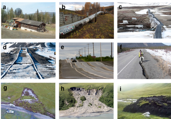
Figure 1 Typical infrastructure damage, geohazards, and thermokarst landscapes related to permafrost thaw. [Images sourced from website]
