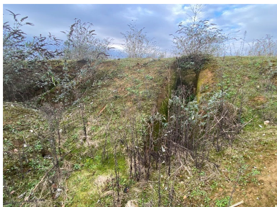
Figure 3. View of the treated embankment in lime-treated soil after 14 years from its construction.
