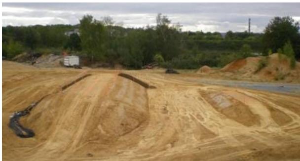
Figure 2. Global view of the two embankments soon after their construction (lime-treated on the left and untreated on the right).
