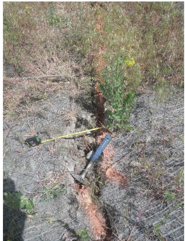
Figure 10. Tension crack at Ripley Slide (post-remediation)
