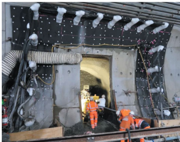
Figure 3. Freeze pipe layout (CP4 as built) and photograph during excavation from southbound tunnel, showing black insulation tiles and ice formed on the freeze pipes.
