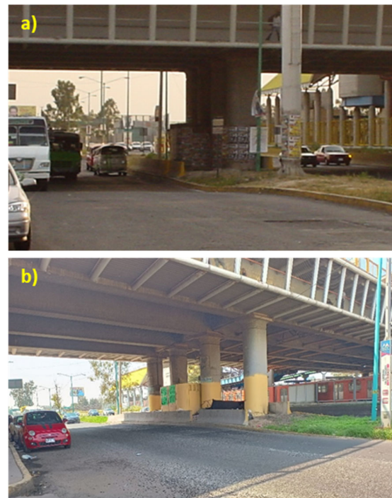
Figure 7. Medium-term settlement and long-term emersion in a piled box foundation in Mexico City.
