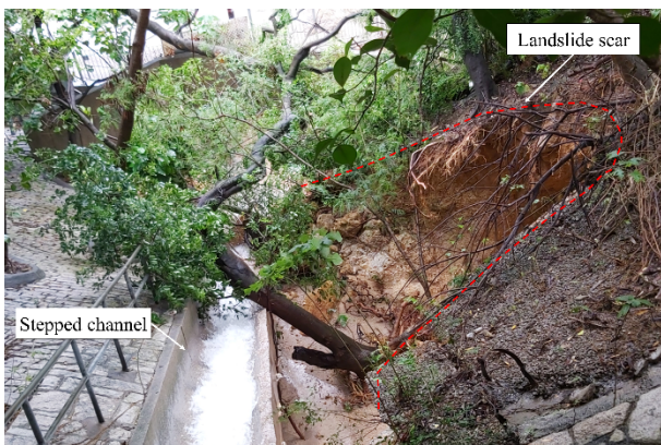
Figure 2. Landslide scar and stepped channel below Wong Tai Sin Road
