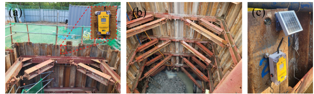
Figure 4. Field deployment of the IoT-based monitoring system at a small-scale excavation site: (a) smart sensor device installed on the earth-retaining wall, (b) overview of the excavation site with installed strut system, and (c) smart monitoring system with solar panel mounted on the retaining structure.
