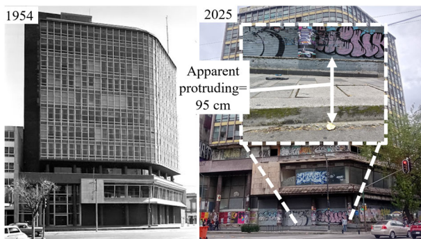
Figure 1. Apparent protruding of a foundation with friction piles.
