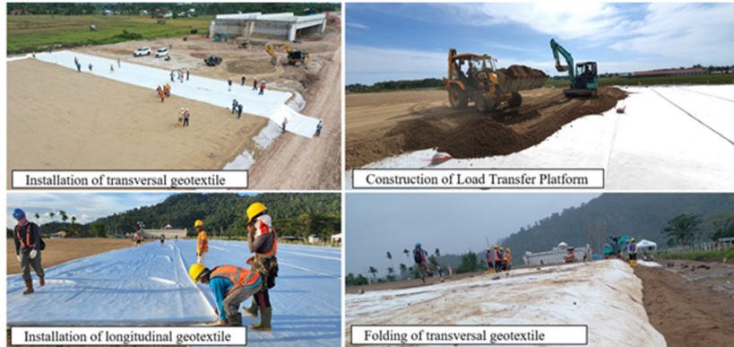
Figure 3. Geotextile installation and LTP construction as part of trial embankment (Himawan et al., 2024).
