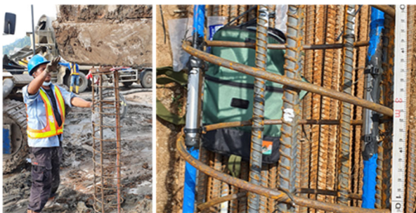
Figure 5. VWSG sensors in the reinforced IKM columns (Himawan et al., 2024).
