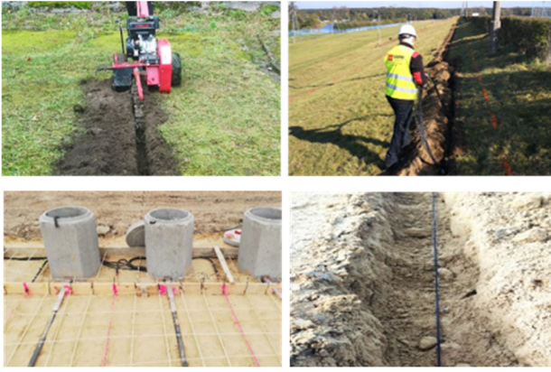
Figure 5. Example installations in earth structures (in wide excavation, narrow trench, sensors end protected in concrete well).
