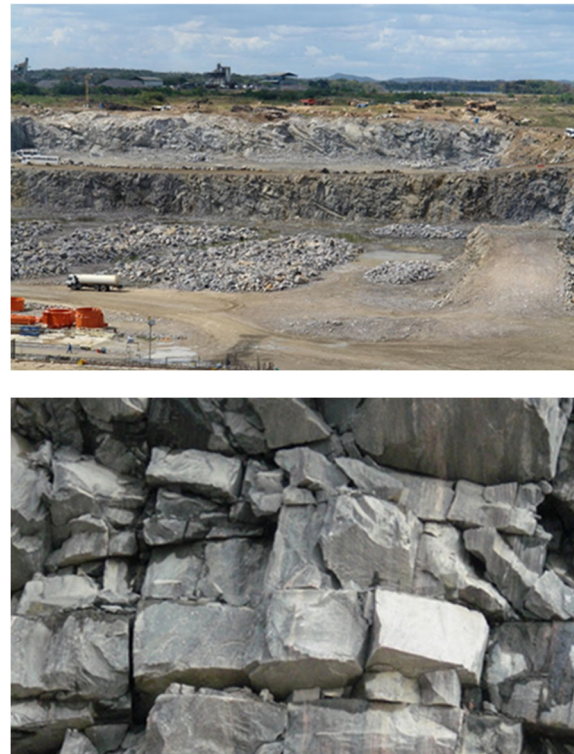
Figure 5. Top: Excavation of the Tocoma Dam spillway channel (Bolívar State, Venezuela). Bottom: Close-up of an excavation face showing horizontal fracture planes delimiting vertical joint patterns.
