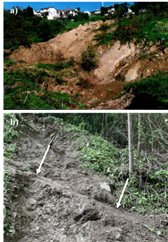
Figure 2. a) Crown of the 1998 soil slide-flow, close to the village of Sedilis. b) Major scarp formed as a result of the 1998 slide showing a pre-existing sliding surface within the colluvial deposit (white arrows).
