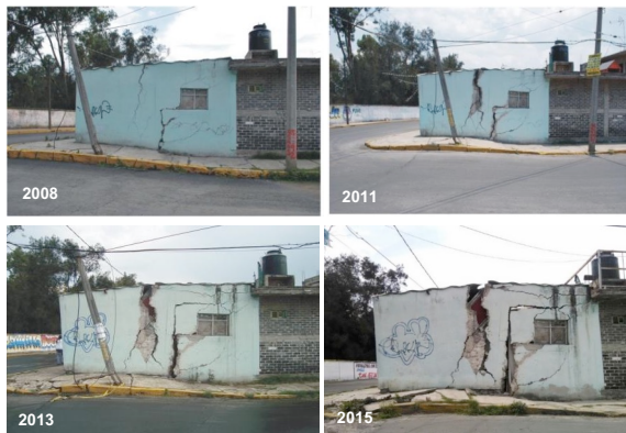
Figure 8. Damage to a house caused by the development of cracking, San Sebastián Tecoloxtitla, Iztapalapa Municipality (SCER, 2024).
