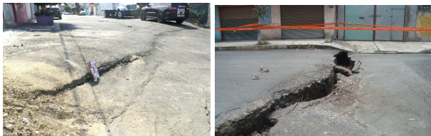
Figure 7. Damages caused to pavements by soil cracks.
