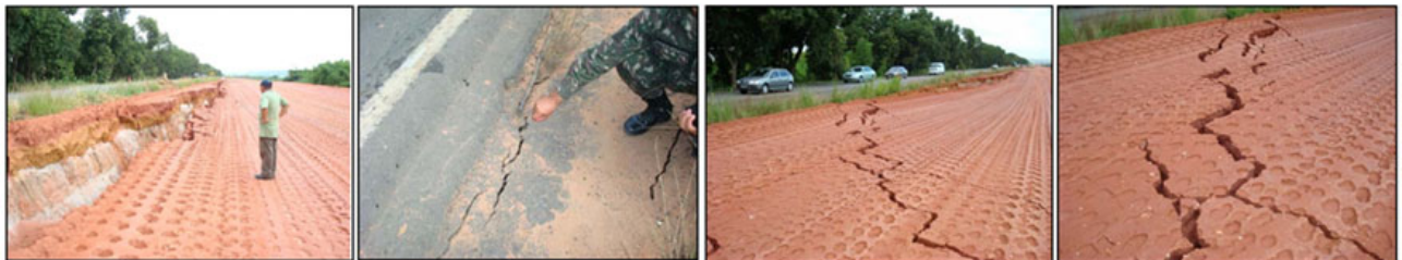
Figure 1. General view of the failure in Embankment 5
