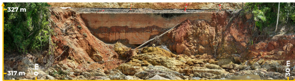
Figure 4. Ground-based photograph of the affected section of the downslope embankment and adjacent linear alignment.
