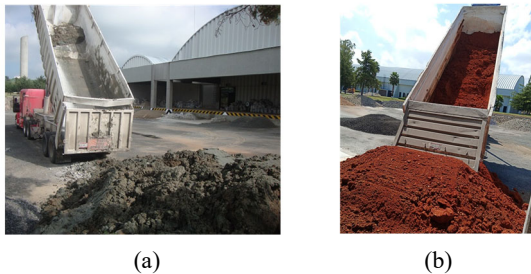
Figure 3. (a) Soil sampled near Lago Chapala, Guadalajara, Mexico; (b) soil 1 of Tren Maya project.
