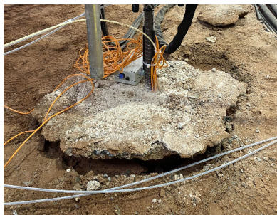
Figure 10. Lack of surface cracks during exhuming a bentonite pile
