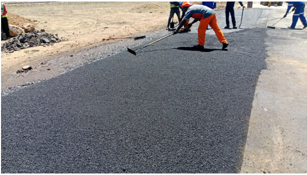
Figure 8. EPWP learners applying and levelling a fresh asphalt layer during road surfacing operations.
