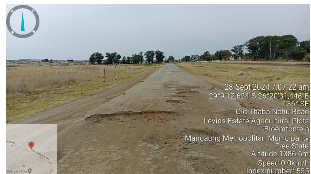
Figure 2. Pavement failure of the A56
