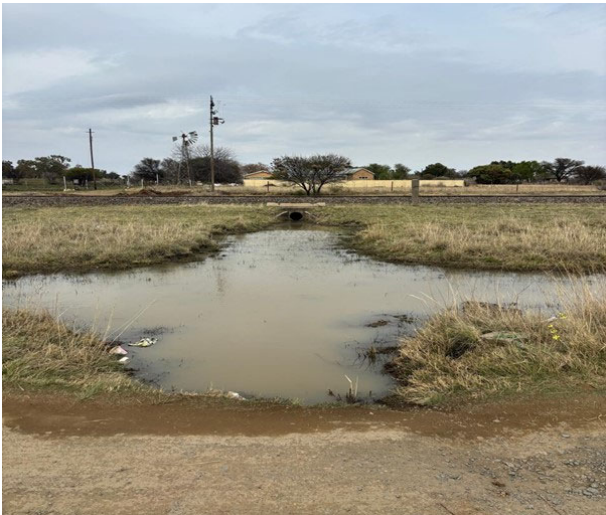
Figure 7. Blocked drain, pooling water and overgrown vegetation.
