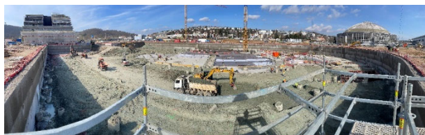
Figure 9. Panoramic view of the completed retaining structure at the start of concreting the foundation slab
