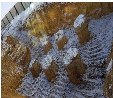
a – Pile cap supported by four bored piles; b – Pile cap supported by six bored piles
